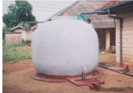
Above ground tank
